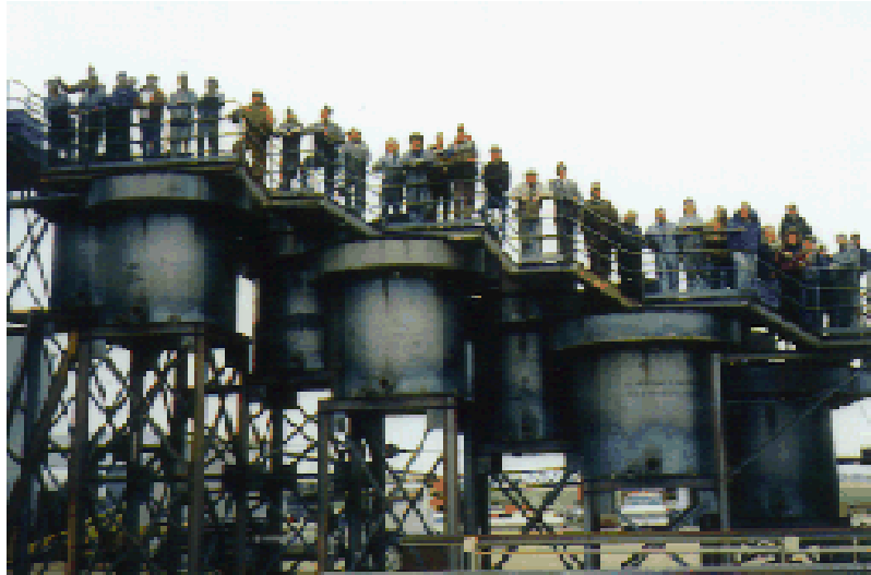
1000 GPM CARBON COLUMN SYSTEM
